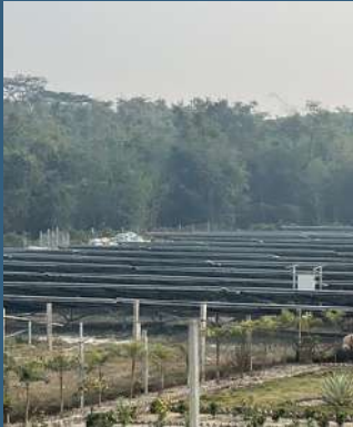
JHAPA SOLAR (12 MW)
