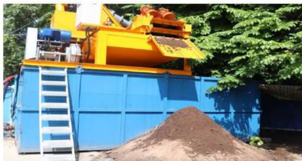
Slurry de-sander system
